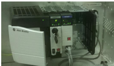
Figure 3: Allen-Bradley ControlLogix controller
